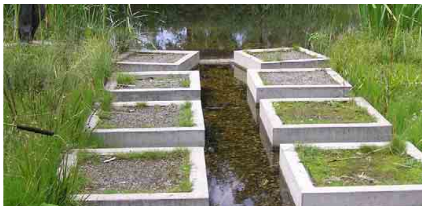
Figure 52. The inlet to the “delta pond” at the downstream end of the Central Drainage Corridor
