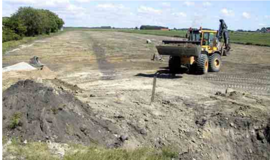
Figure 75. The construction work is starting at the downstream end of the eastern part of the Fjärilsparken Eco-Corridor.
